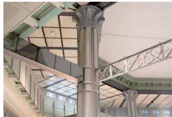
丸の内南口ドーム竣工写真 Perspective view of the structure below completed dome ceiling at the Marunouchi South Entrance
