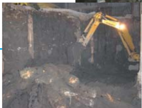
(上) 地上に近い階から施工 (下) 松杭を少しずつ撤去 (Above) Carried out from floor closest to surface (Below) Pine stakes removed one by one
