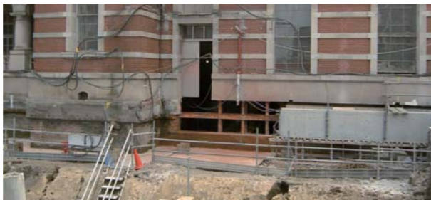
免震化計画 縦梁の構築状況 Seismic Beam Isolation Plan Vertical Beam Construction Status
